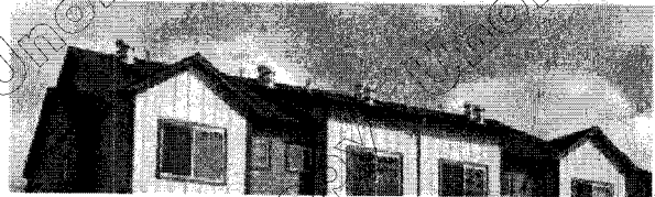
Mechanical vents reflect architectural style
