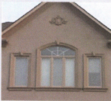
NOT PERMITTED: stucco pop out
